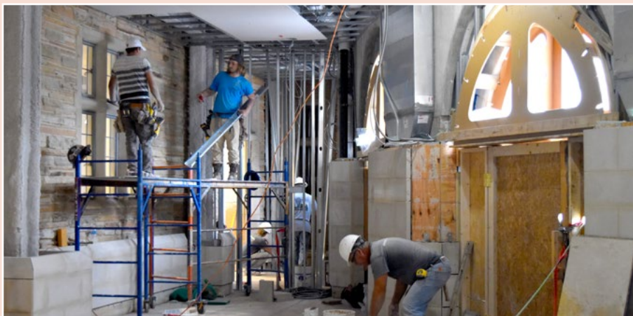
The interior is abuzz with activity in every area — each worker doing his part within a team: ceilings, archways, staircases, door installations, drywall, finishing ... it won't be long until Grand Opening!
